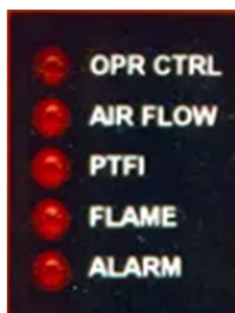
Figure 8: Relais de surveillance de flamme (FIREYE)
