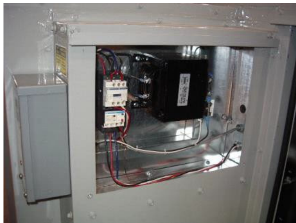
FIGURE 2: Electrical connection and high voltage disconnect.
